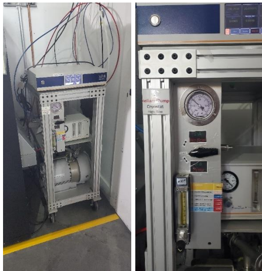
Figure 11: Evacuation pump and helium fill station behind the outboard hutch door at BioXAS-Side.
