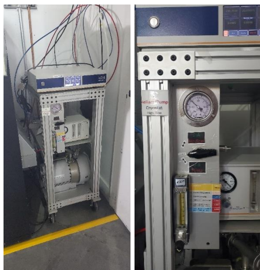
Figure 11: Evacuation pump and helium fill station behind the outboard hutch door at BioXAS-Main.
